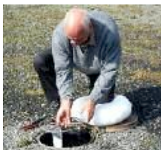
3. Lower the meter system back into the pit, turning the wheel slightly as it goes.
